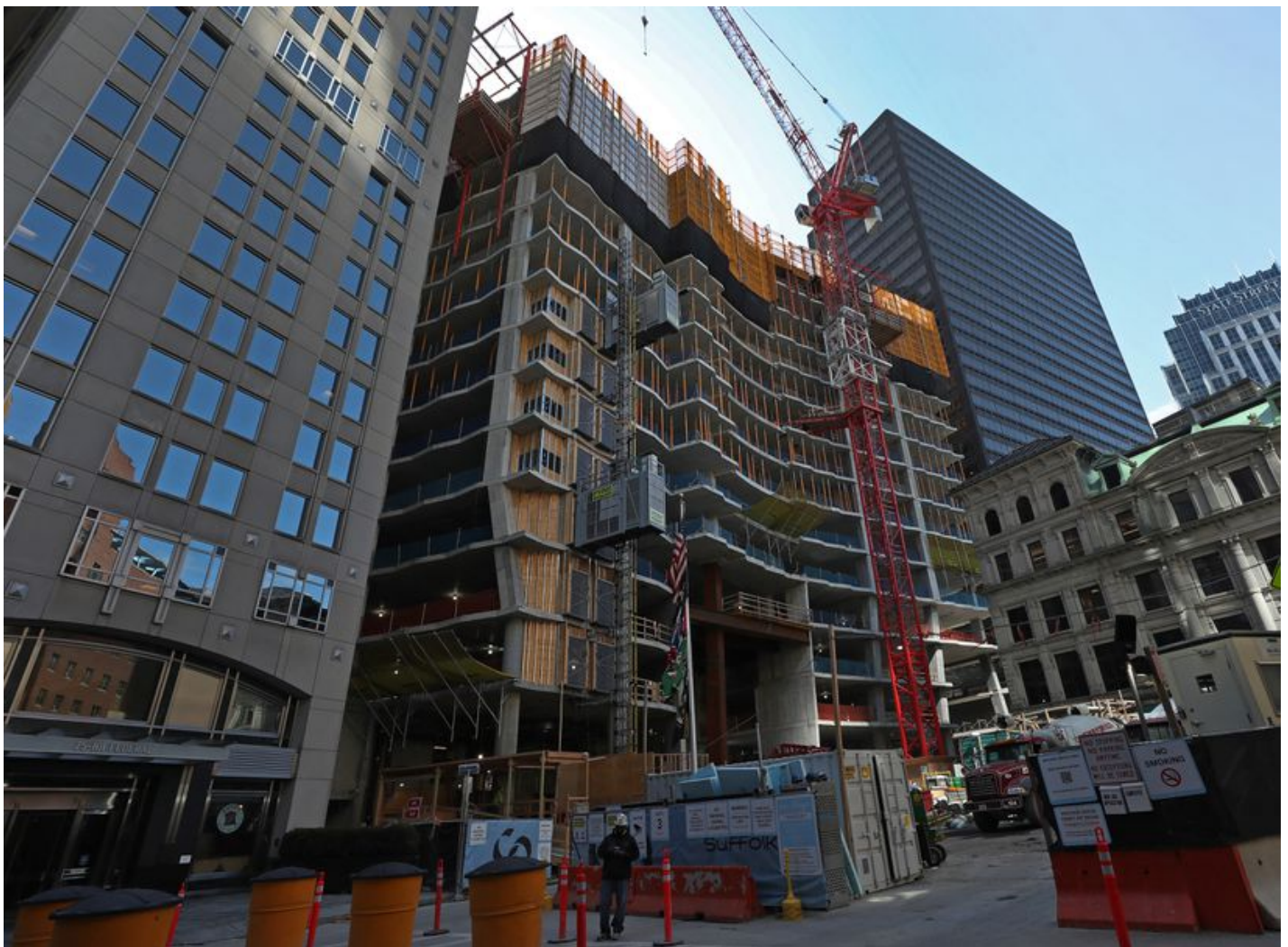
Construction in April 2021 on the Winthrop Center tower on Devonshire Street downtown. DAVID L. RYAN/GLOBE STAFF
