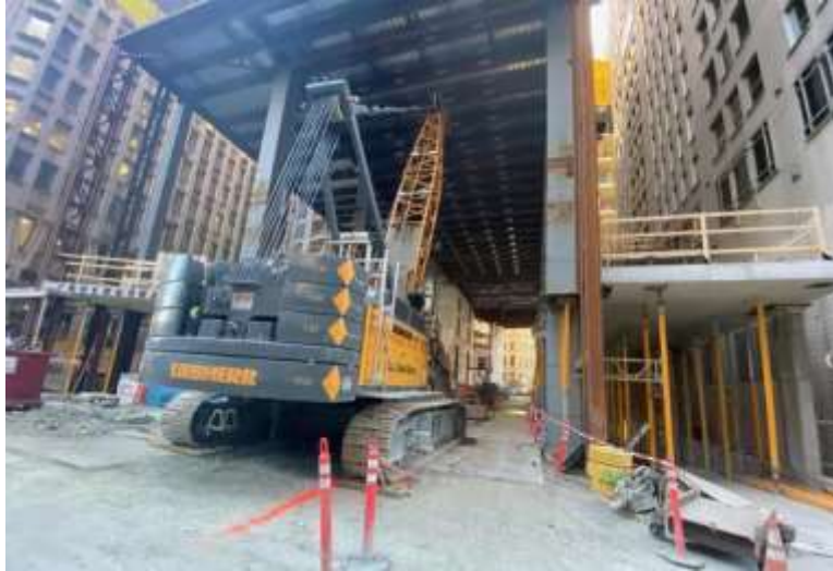
A crane parked underneath the roof of The Connector at Winthrop Center.
